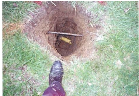
Exposed Services in Pot-Hole
